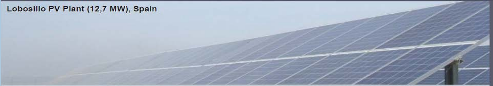
Lobosillo PV Plant (12,7 MW), Spain
